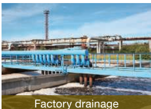
Factory drainage For monitoring final discharge water
