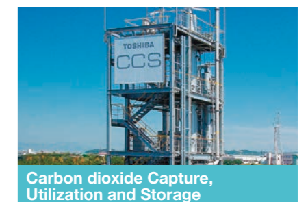
Photo: CO 2 separation and capture equipment. Courtesy of Toshiba Energy Systems & Solutions Corporation
