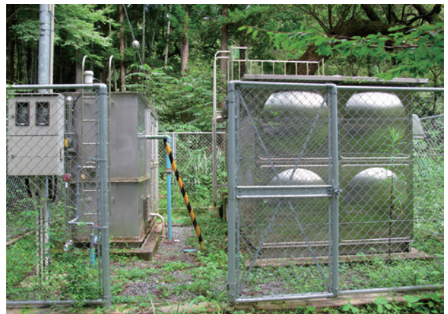
Photo 1 Water supply facility installed in Hamamatsu City, Shizuoka Prefecture
