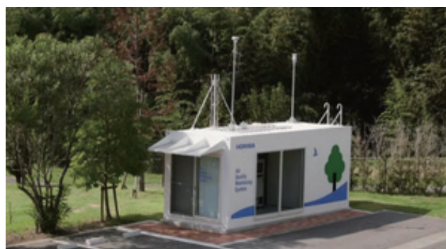
Figure 5 Air Quality Monitoring Station (AQMS)
