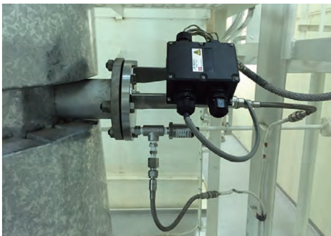
Figure 13 MEXA-820NO x arranged in the front and the rear of SCR
