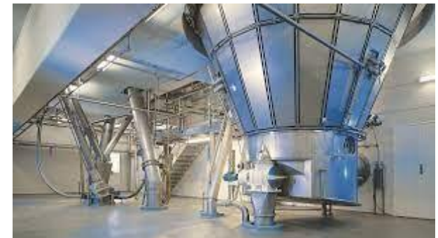
Production Tower Dryer
