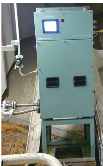
Figure 5 Installation on board
